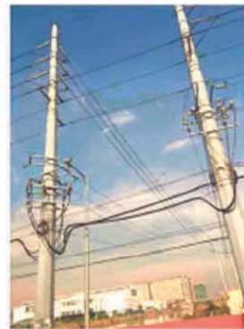
138KV电力杆 138kv power pole
