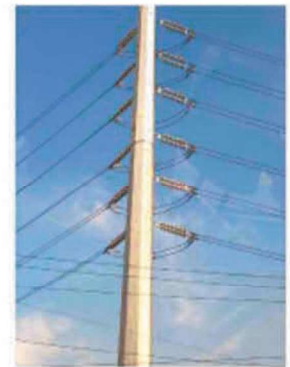
转角电力杆 Angle power pole
