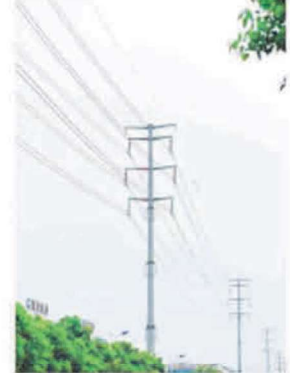
直线电力杆 Straight power pole
