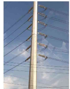
转角电力杆 Angle power pole
