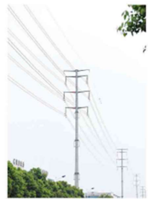
直线电力杆 Straight power pole
