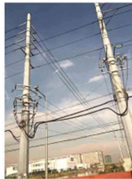
138KV电力杆 138Kv power pole
